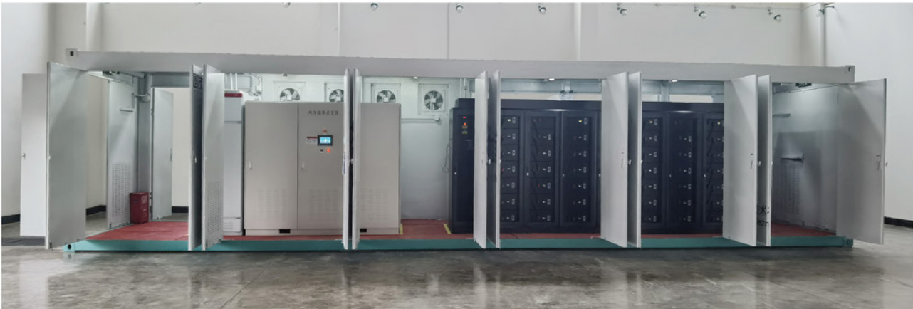
▼ 500KW Lithium phosphate battery energy storage system Zibo, Shandong
